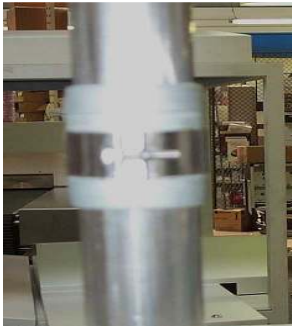
Figure 7.7. Exhaust Stack Heater
