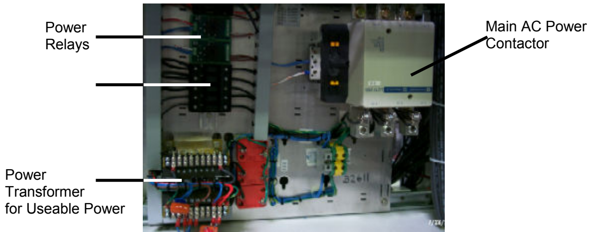
Figure 3-6: Safety Enclosure Panel
