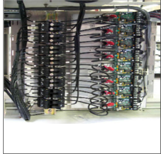
Figure 3-5: SCR Panel & fuses
