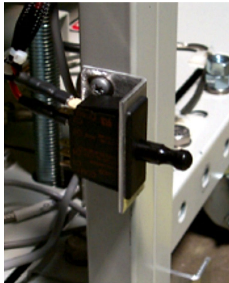
Figure 2-2: Panel Switch Installed Override Mode Position
