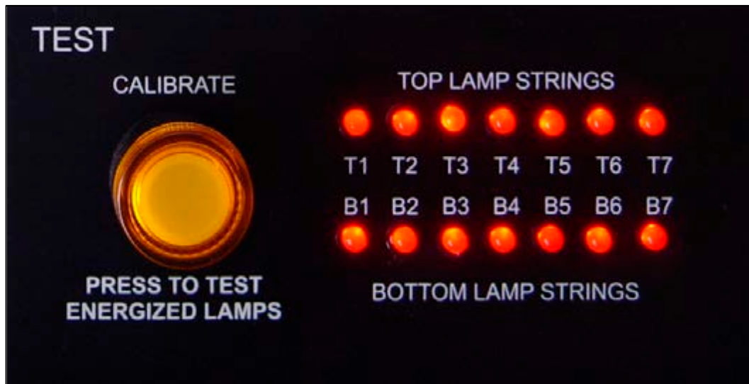
Figure 7-13 Test Panel: Lamp String Failure Indicator
