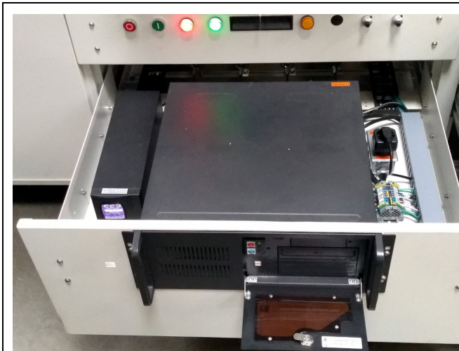
Figure 1-50 Factory UPS (left)
