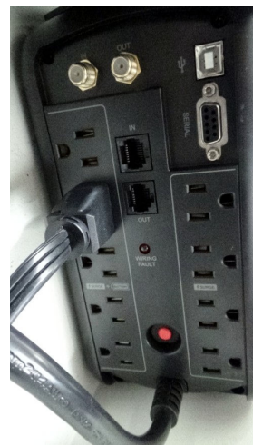
Figure 1-51 UPS, rear view
