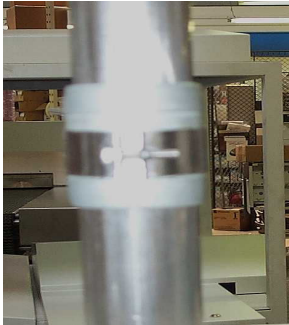
Figure 7.7. Exhaust Stack Heater
