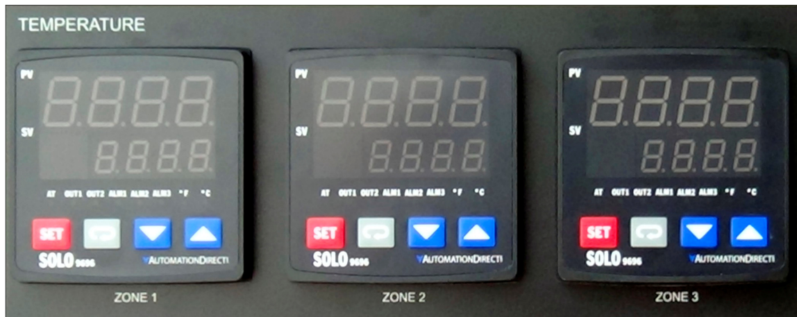
Figure 1-13 Zone Temperature Controllers
