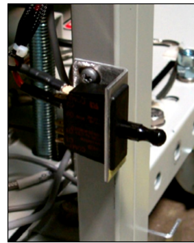
Panel Switch Installed - Bypass (out) Position
