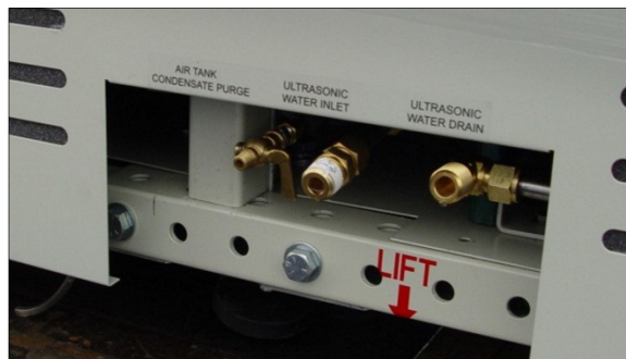
Figure 2-31 UCD Water Connections with Air Purge
