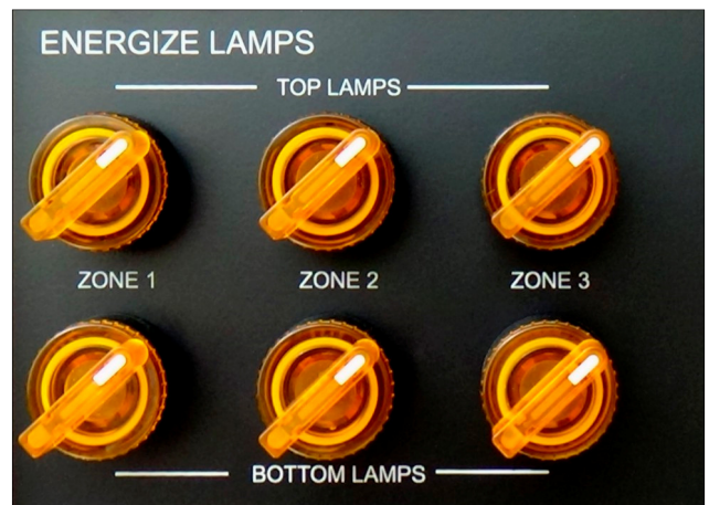
Figure 1-12 Energize Lamps control panel
