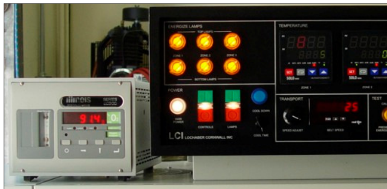
Figure 6-11 Oxygen Analyzer next to Control Console
