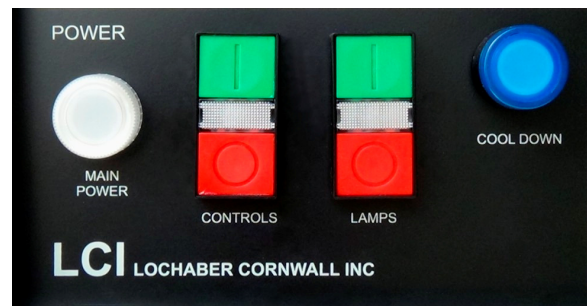
Figure 1-11 Power control panel
