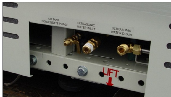
Figure 2-30 UCD Water Connections with Air Purge
