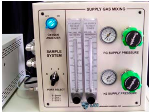
Figure 6-13 Sample System control panel (shown with Supply Gas Mixing System)
