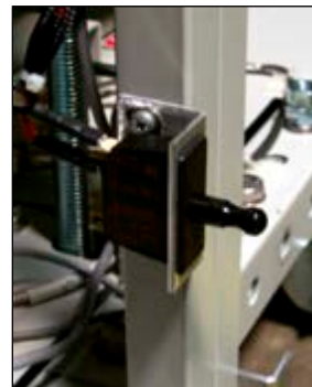
Panel Switch Installed - Bypass (out) Position
