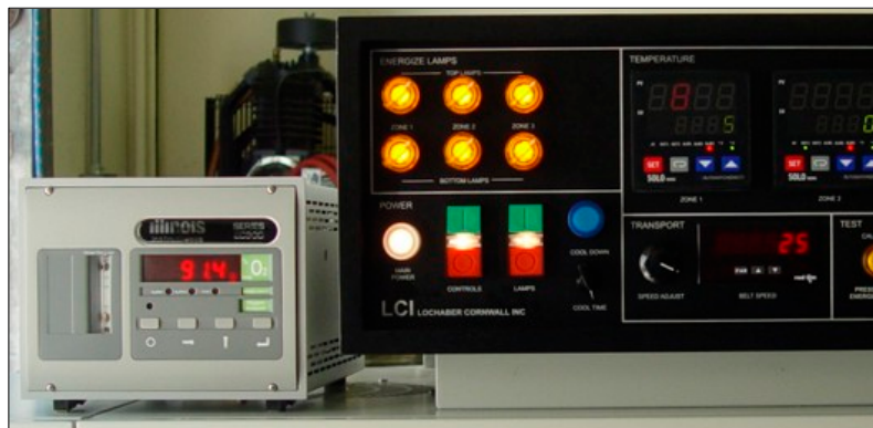
Figure 6-11 Oxygen Analyzer next to Control Console
