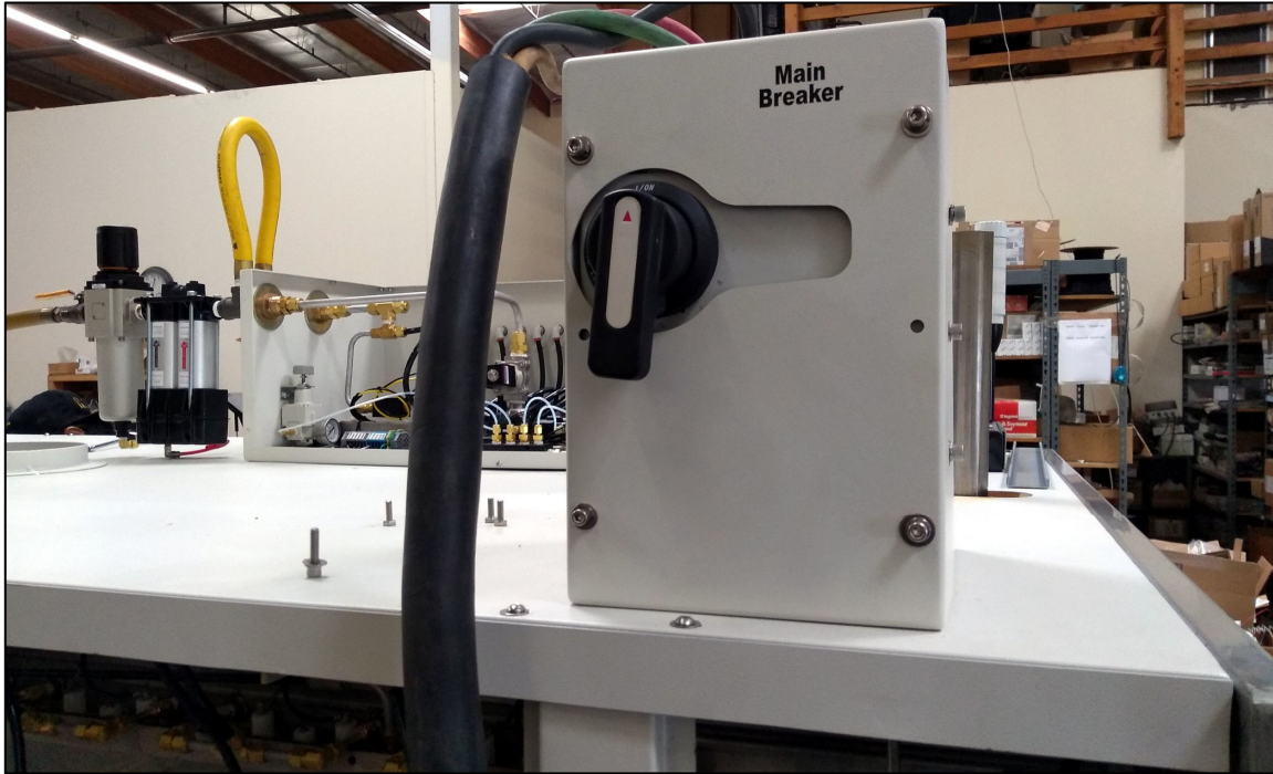
Figure 2-20 Top mount circuit breaker
