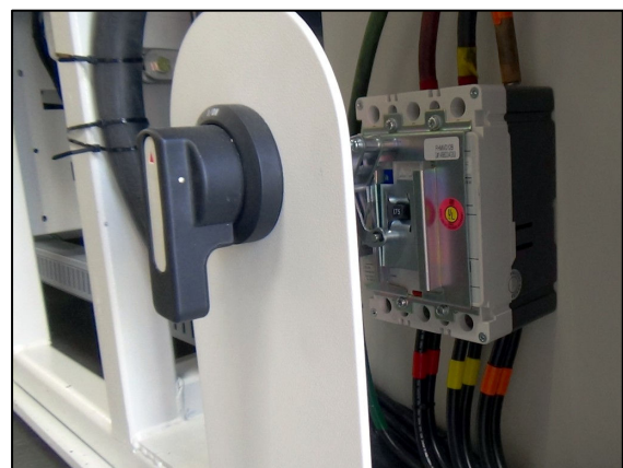
Figure 2-19 Disconnect switch & power connection terminal blocks
