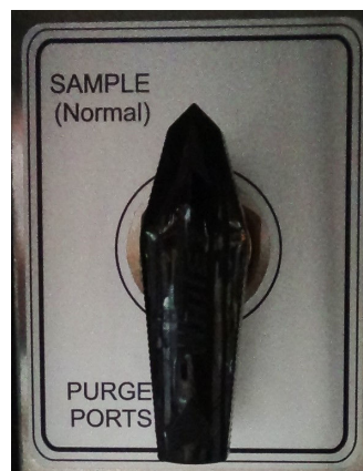
Figure 4-23 Sample-Purge valve on OSS panel
