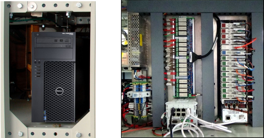
Figure 4-17 Computer and UPS (L) PLC panel (R)
