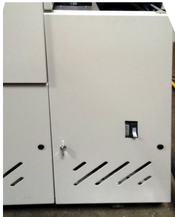
Figure 2-19 Circuit Breaker panel
