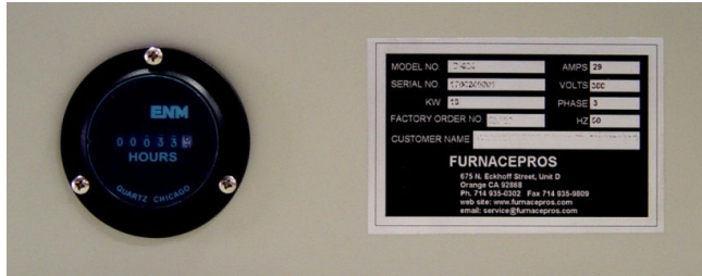
Figure 2-17 Elapsed Time Meter and Nameplate
