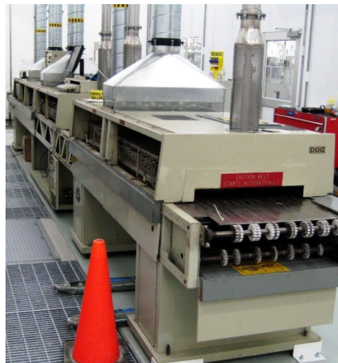
Figure 2-33 Cabinet Exhaust Examples
