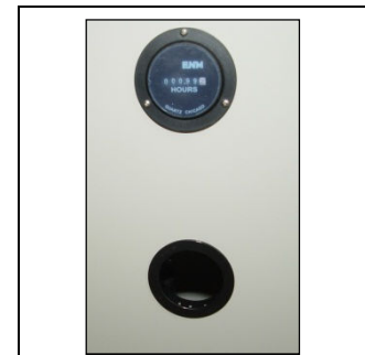
Figure 2-15 Standard Front Entry Power Port and Elapsed Time Meter
