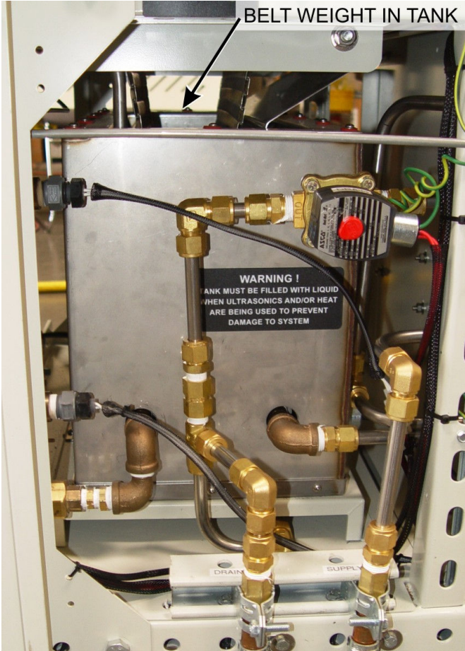
Figure 2-14 Belt weight in Tank on UCD system
