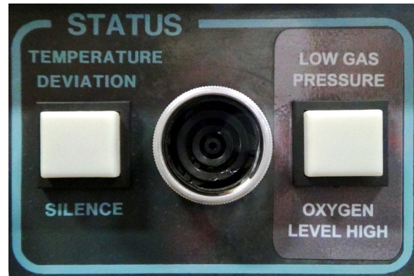
Figure 1-12 Status Panel and Alarm Controls
