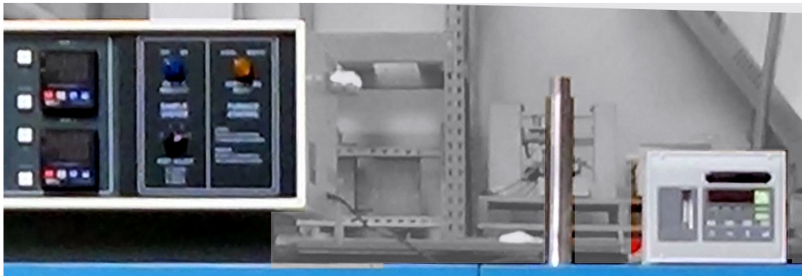
Figure 1-37 Oxygen analyzer next to OSS sample system
