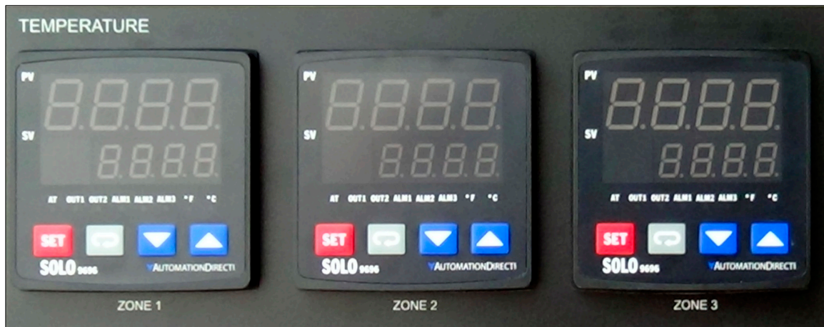
Figure 1-18 Zone Temperature Controllers
