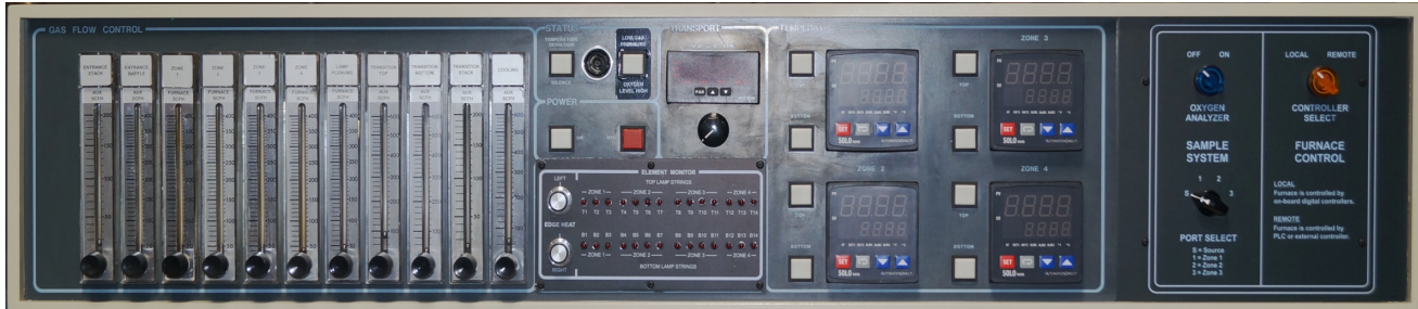
Figure 1-10 Furnace Control Console
