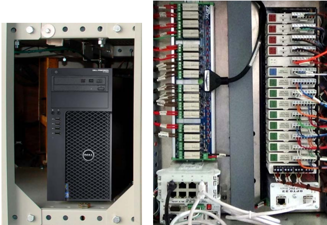
Figure 0-11 Furnace Computer (L) and PLC Controller (R)
