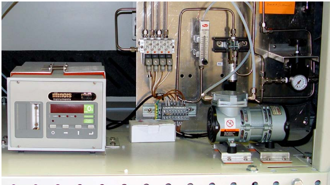
Figure 0-27 Oxygen analyzer next to OSS sample system
