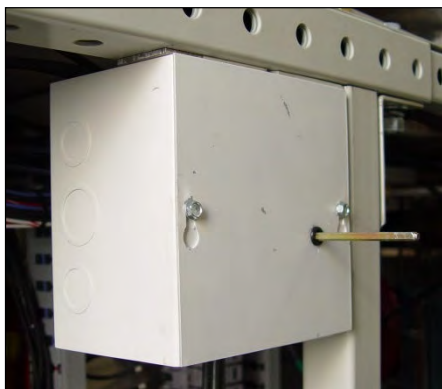
Figure 1.2.7 Disconnect Switch Enclosure
