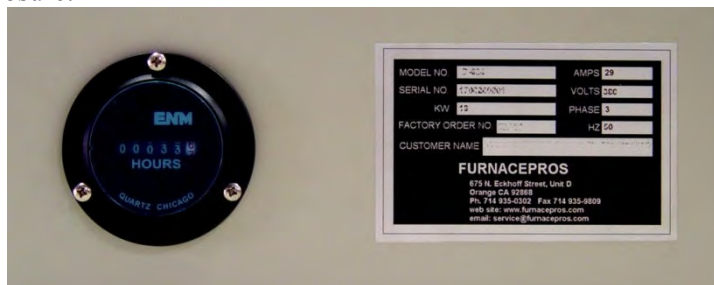
Figure 1.2.6 Elapsed Time Meter and Nameplate
