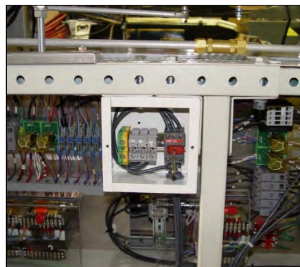
Figure 1.2.8 Enclosure Cover Removed
