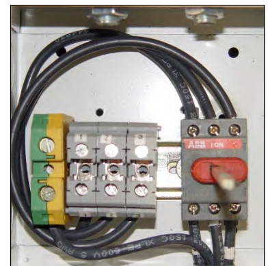
Figure 1.2.9 Disconnect Switch and Power Connection Terminal Blocks
